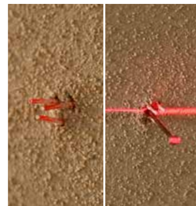
Elastic projection to permanently ensure surveyed measurements are securely marked until after plastering work.
