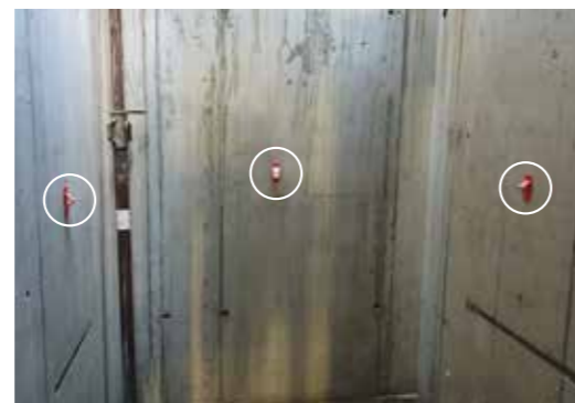
RSAK130 mounted on axis in a lift shaft.
