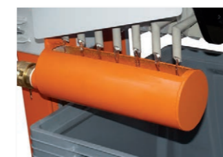
Filter outlet with drain gutter
