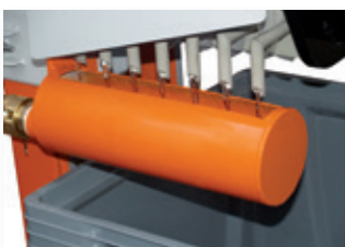
Filter outlet with drain gutter
